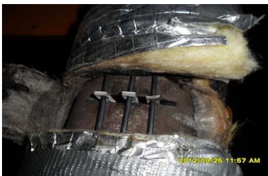
Fig.1. The placing of the samples in the exhaust pipe of the AV00 boiler
